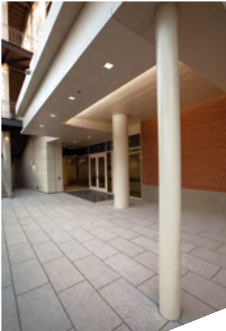
4-inch, square ceramic metal halide downlights illuminate this portico, connecting lecture halls of a major university.
